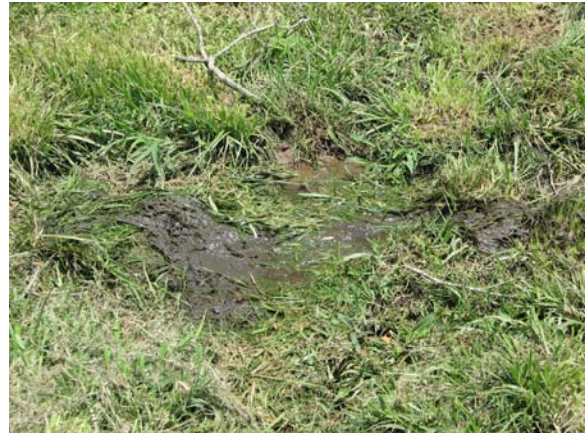
On ground sewage resulting from failed septic tank.
