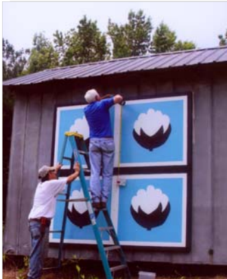
Council Member, Denney Rogers, installing Cotton Ball Quilt on barn in Heard County
